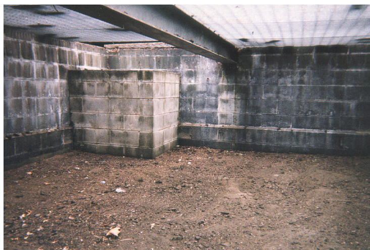
Figure 6.2. Underground sand filter for a car park in Auckland, New Zealand
