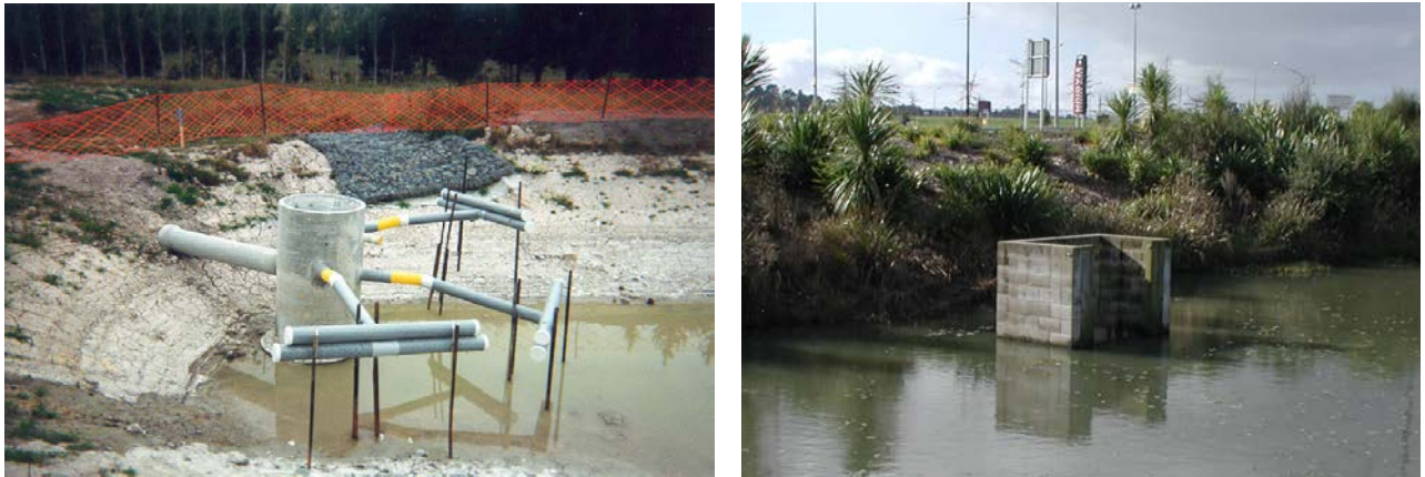
Figure 3.6. Sedimentation Basin Outlet Structures (L) a floating skimmer and (R) a narrow weir
