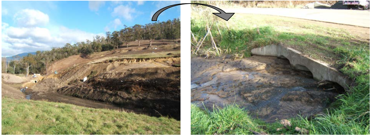
Figure F-1. Unmanaged runoff from this construction site has resulted in blocked stormwater infrastructure and heavy siltation in the nearby creek.
